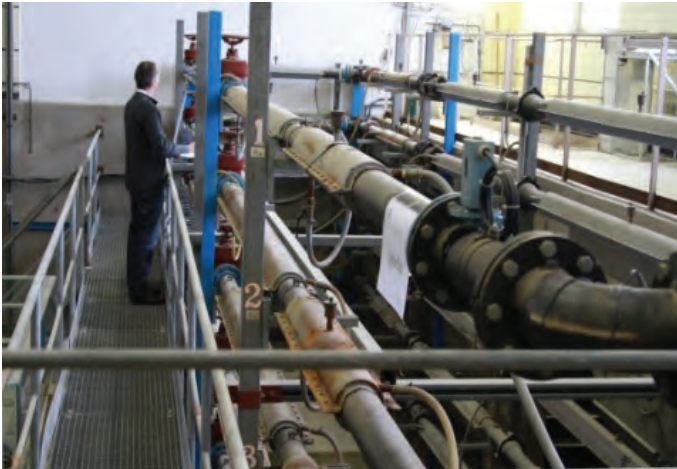
Figure 3: Water Treatment Plant of the City of Nancy in France
