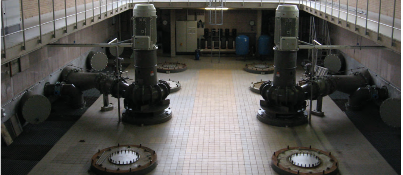
Figure 6: Pumps in Water Treatment Plant of the City of Amsterdam
