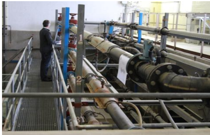
Figure 3 Drinking water pilot plant made of several loop serially disposed
